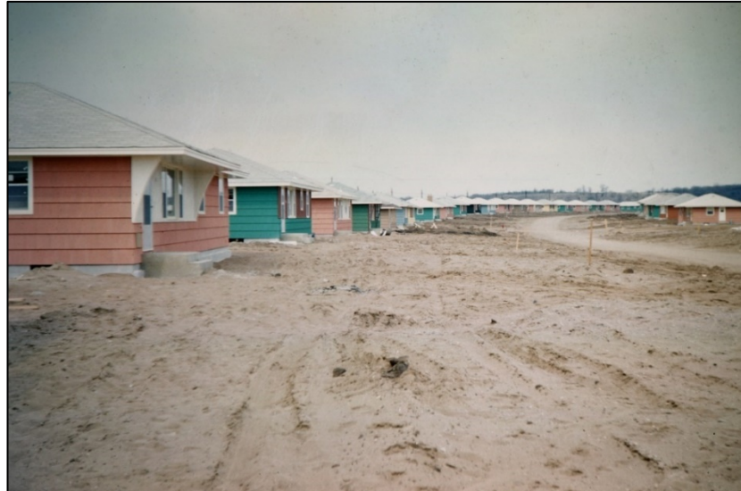
Figure 3.3. Ranch houses under construction in the 8500 block of Greenway Avenue South within Thompson Grove, ca. 1960. Image courtesy of Tony Brinkman.
