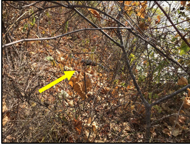
Location 3 – drain tile at surface on bank
