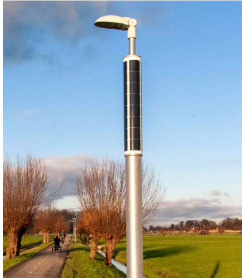
Soluxio Smart Solar Wireless Access Point with Street Light
