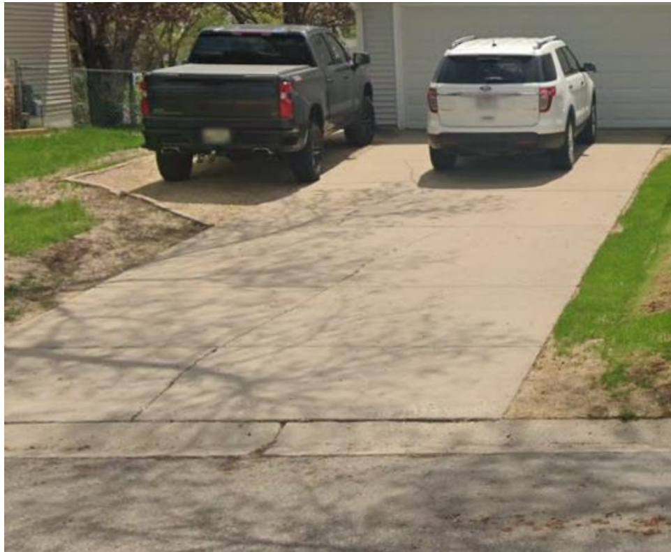
Example of a non-conforming Class 5 driveway that could be improved.
