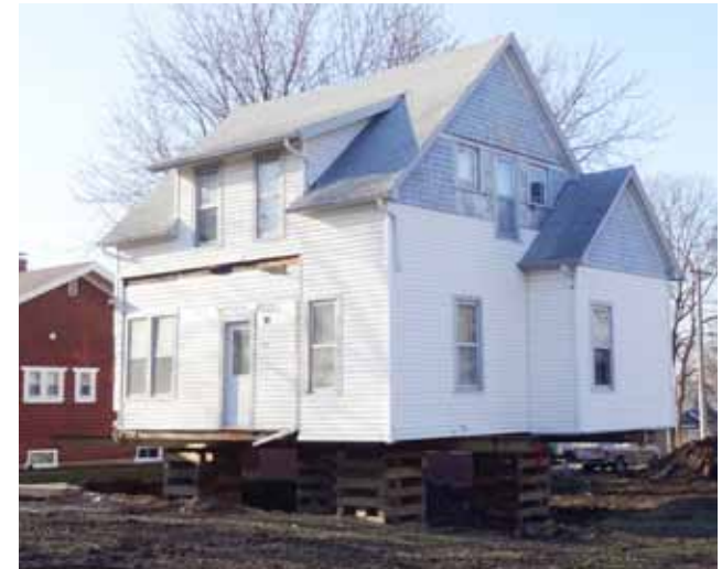
This residence is undergoing a foundation and porch alteration. A project of this degree requires thorough review.
